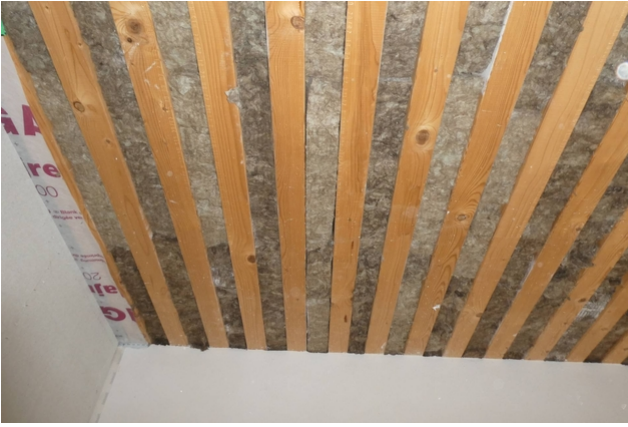
Ceiling insulation in barn conversion
